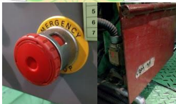
Figure 5.2 Button & Kick Plate Emergency Stop
