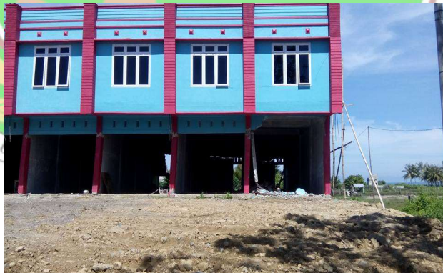
Gambar 1.5 Bangunan Ruko Mengalami Soft Story di Kab.Pidie Jaya ( Sumber :ft.blogspot.com/2016/12/soft-story-effect-pada-musibah-gempa.html)
