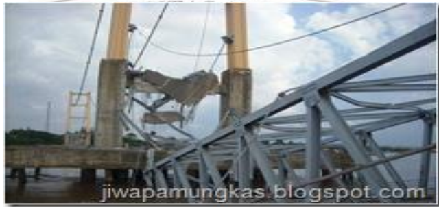
Gambar 1.2 keruntuhan Jembatan Mahakam 2, Kaltim
