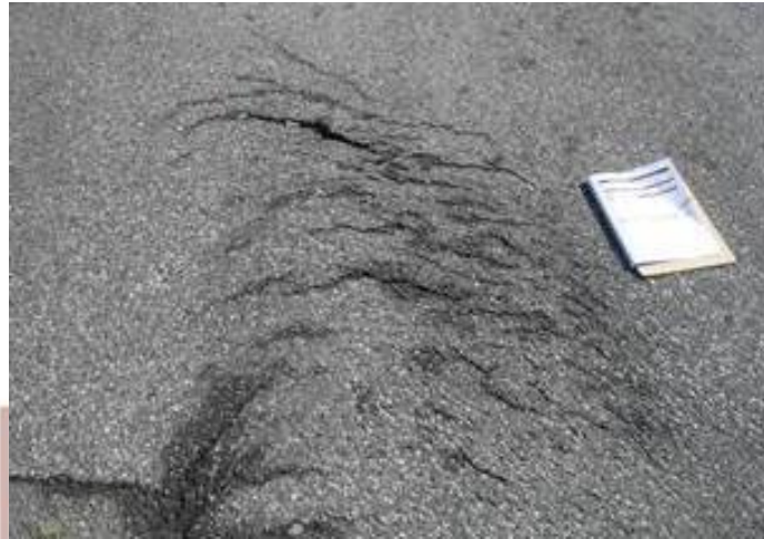
Gambar 1.10 Retak Slip (Slippage Cracks)
