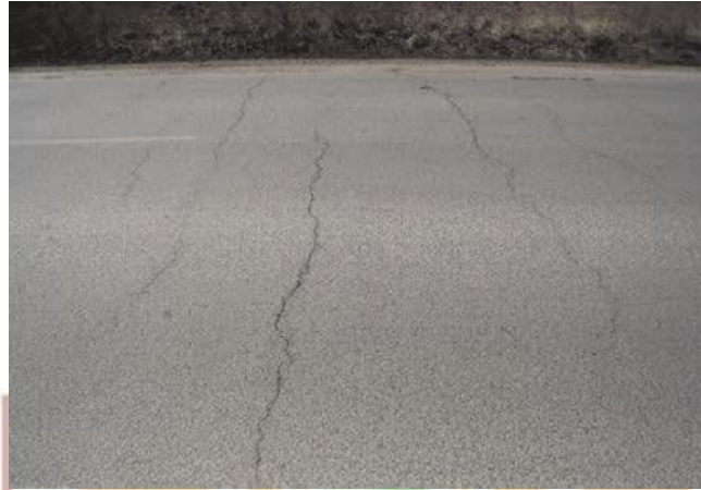
Gambar 1.6 Retak Melintang (Transverse Crack)
