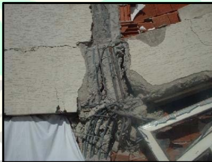
Gambar 1.2 Kegagalan Balok-Kolom Joint
